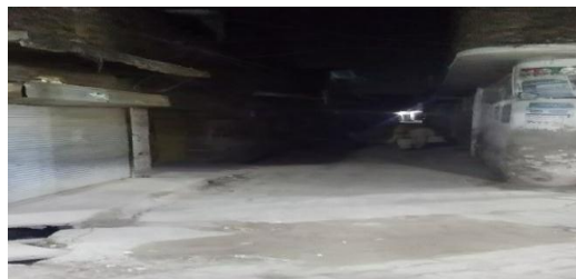
No streetlight by TMA
